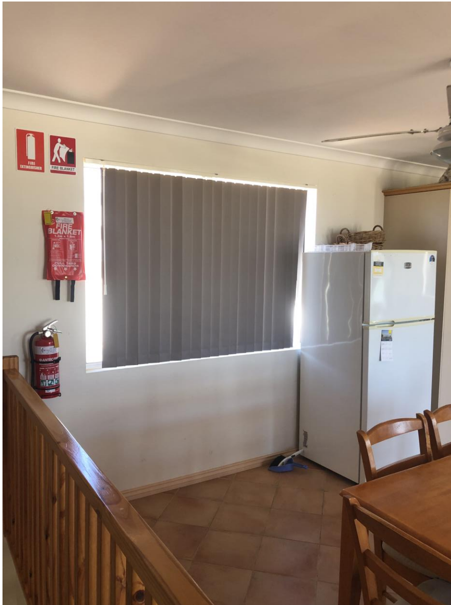
Fire Extinguisher and Fire Blanket - upstairs
