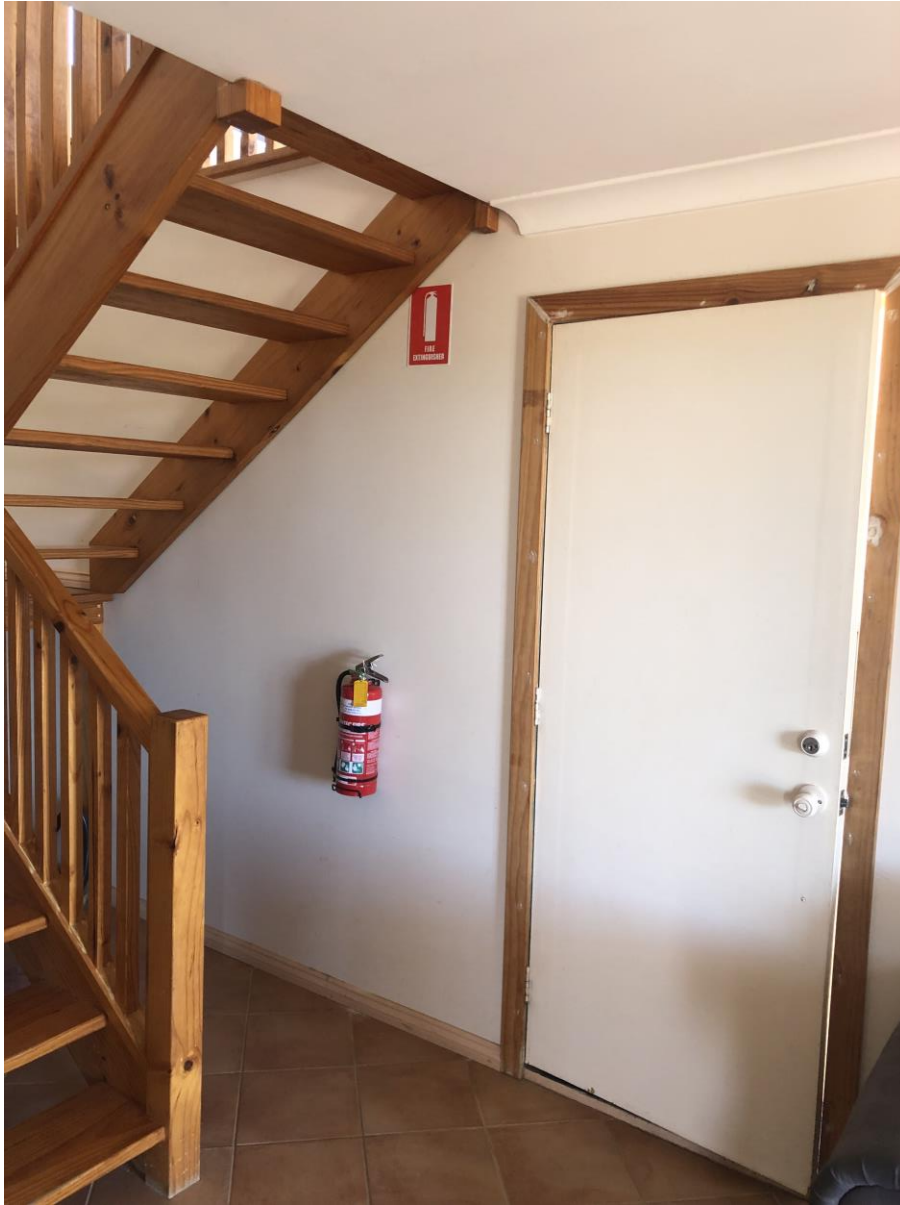
Fire Extinguisher - downstairs
