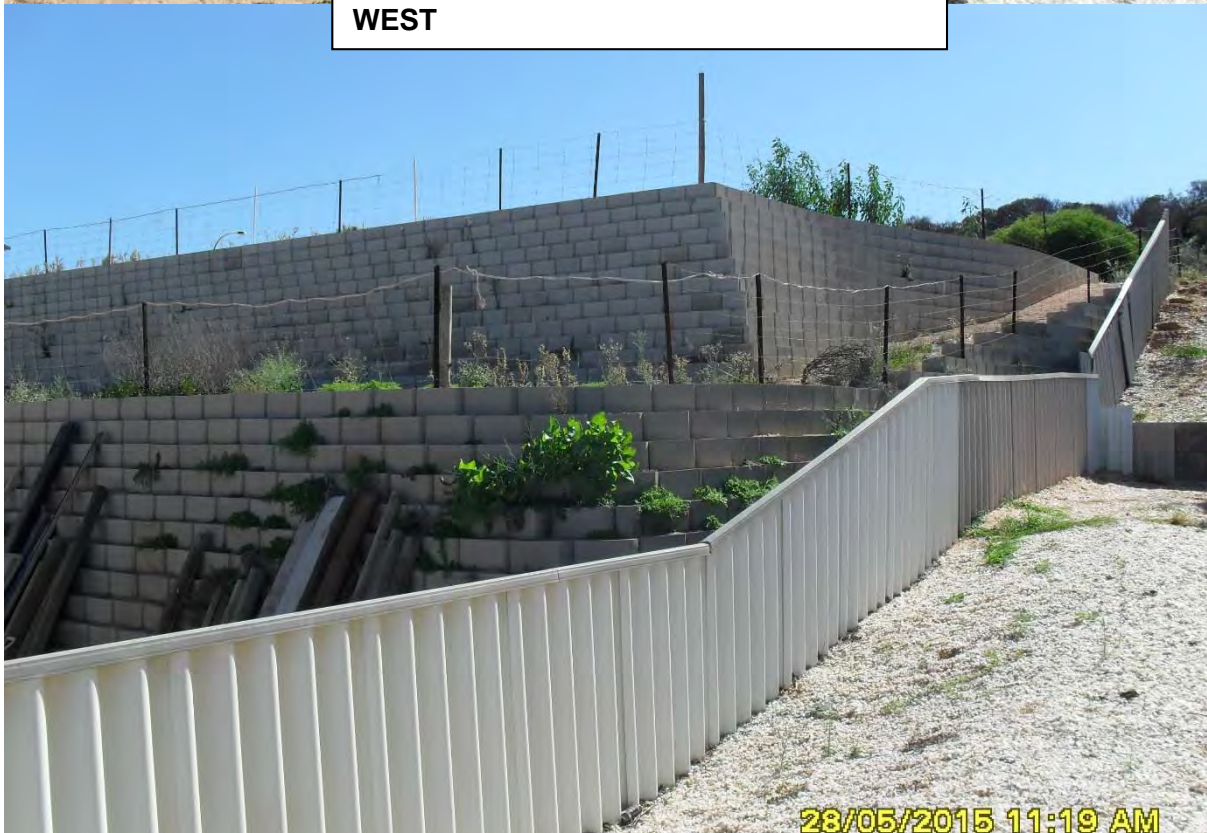
Site Inspection Photographs taken by Glenn Bangay, Principal Environmental Health Officer / Building Surveyor
