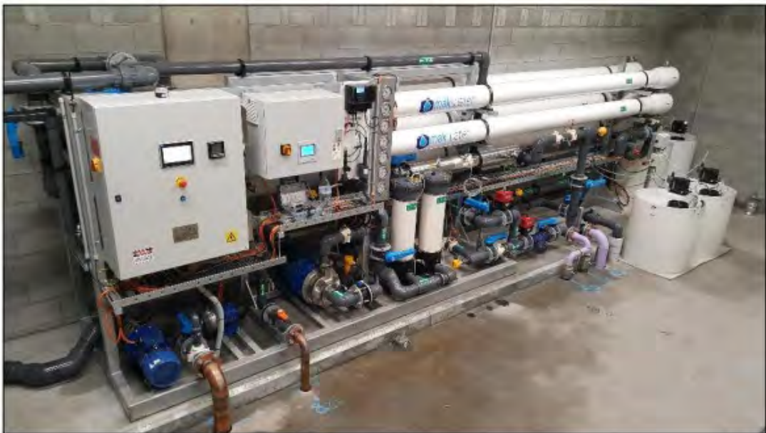
A MAK Water skid mounted RO plant installed onsite
